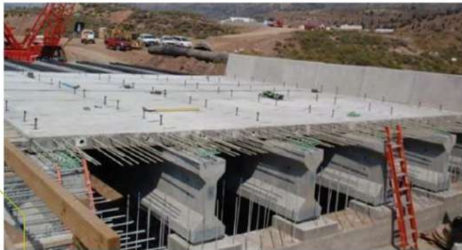
Fig. 3.2d—Emma Park Bridge deck panel with GFRP reinforcing bars, top and bottom mat.
