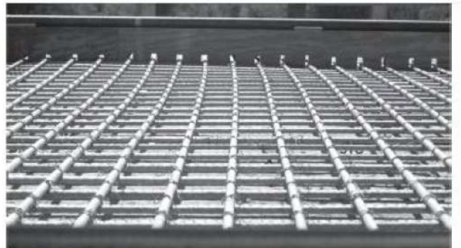
Fig. 3.2c—Transverse view of GFRP bars in Sierrita de la Cruz Creek Bridge deck near Amarillo, TX, in 2000.
